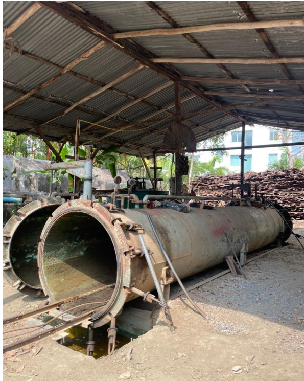
Figure 14: The impregnating tank at the Sanctuary of Truth. The tank uses the pressure process to prolong the lifespan of the wood.
